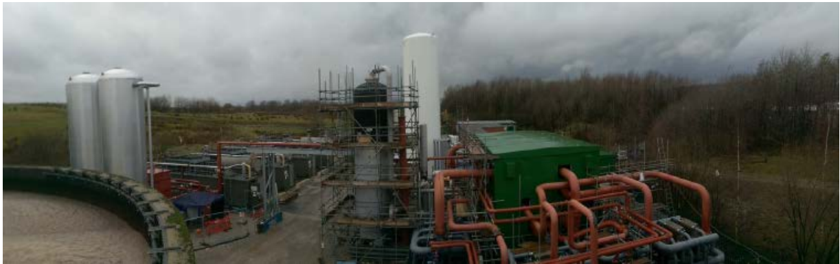
Fig. 3.8. Highview 5MW/15MWh Commercial Demonstration plant in Manchester Integrated with Viridor Biogas Power Plant
