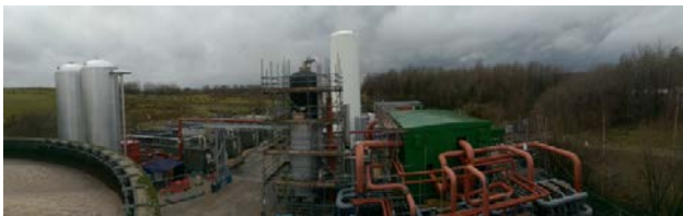
Fig. ES.5. Highview 5MW/15MWh Commercial Cryogenic Demonstration plant in Manchester Integrated with Viridor Biogas Power Plant
