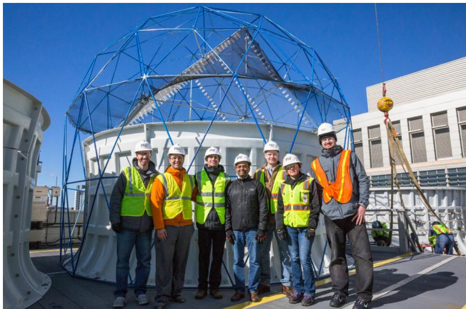
On the Central Utility Plant roof in front of the newly installed water-capture system (from left): Derek Warnick, COO, Infinite Cooling; Karim Khalil PhD '18; Maher Damak PhD '18; Professor Kripa Varanasi of mechanical engineering; Patrick Karalekas, plant engineer, and Jodi Cooksey, safety engineer, Central Utilities Plant; and Erich Ryan, intern, Infinite Cooling. Photo: Kelley Travers, MITEL
