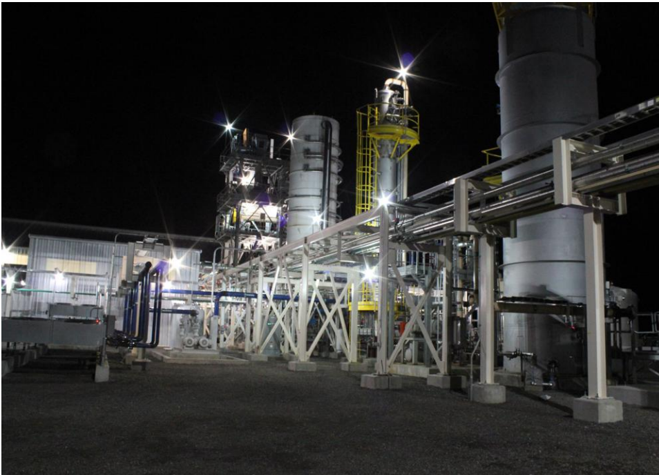
This InEnTec plant in Oregon will receive feedstock materials such as medical and industrial waste and—using InEnTec's plasma gasification process—will convert them into high-purity hydrogen for use in industry and fuel cell vehicles. Photo: Jeffrey E. Surma, InEnTec
